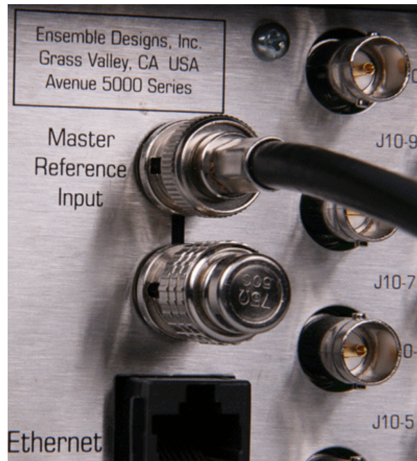
Connecting a Timing Reference to the Master Reference Input on the rear of the Avenue Frame. The loop through is terminated with a 75 ohm termination.
